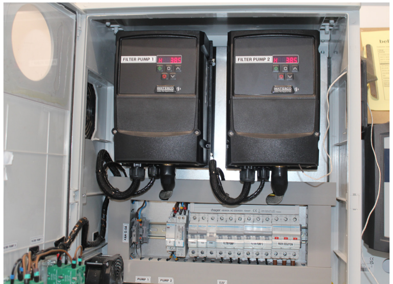
Waterco Variable Frequency Drives are installed to reduce electrical consumption.
