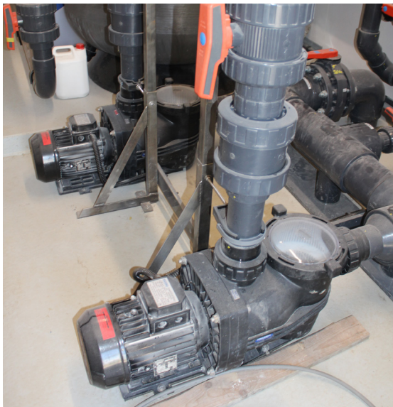
Installed are 2 x Hydrostar 5.5HP commercial pumps for maximum performance and quietness.
