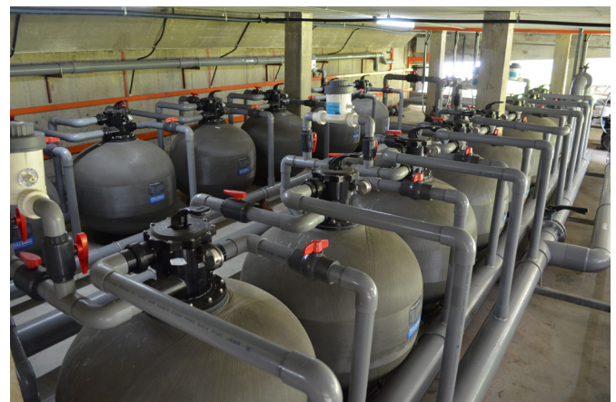
Waterco water filtration system set-up for swimming pools at BKECR
