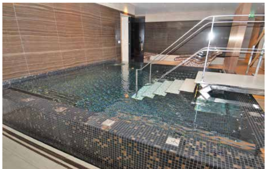
Full-service spa and swimming pool facility fitted with Waterco's commercial pumps and filters.
