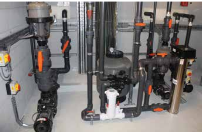
The plantroom for the children's play pool and the cascading waterfall comprising of Micron filters, EcoPure Glass media, multicyclones and the Hydrostorm Pumps.
