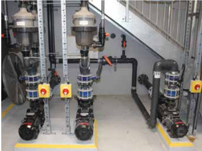
"Waterco's range is terrific and the quality consistently high, which complements the other equipment we use," Nick Roberts explains.
