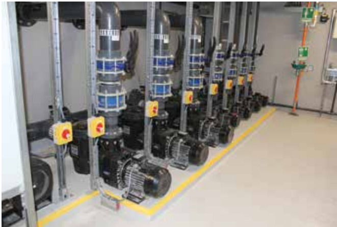
Hydrostar Pumps to power the various water features including the main fountain pool and connecting features
