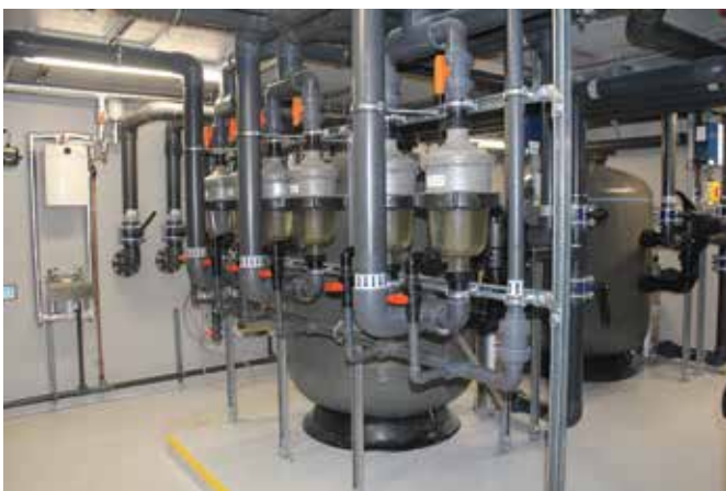
Multiple SMD Commercial Filters and Multicyclones ensures the highest level of water quality for the various water features.
