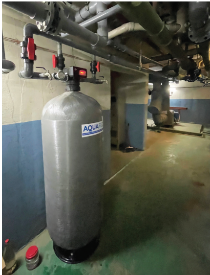
Aquaflo centralised water filtration system installed in the basement of Menara Chan.
