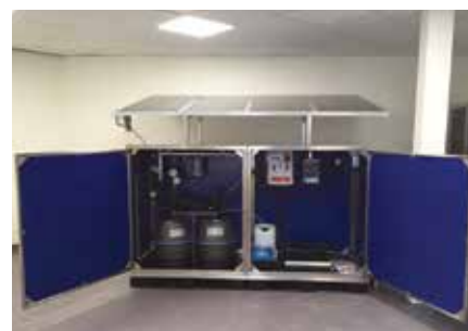
Each system consisted of a solar pump, a T400 filter with glass pearl media and T400 filter filled with activated carbon, a UV sterilizer, a chlorine dosing pump.
