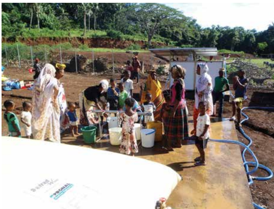
▲ Sotrad Water needed to come up with a robust and affordable system that pumped water from the available sources such as streams, open wells, boreholes or lakes.
