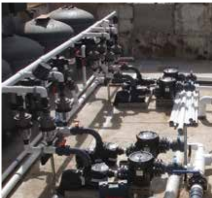
Eight MultiCyclones plus six Micron SMD deep bed fiberglass media filters.
