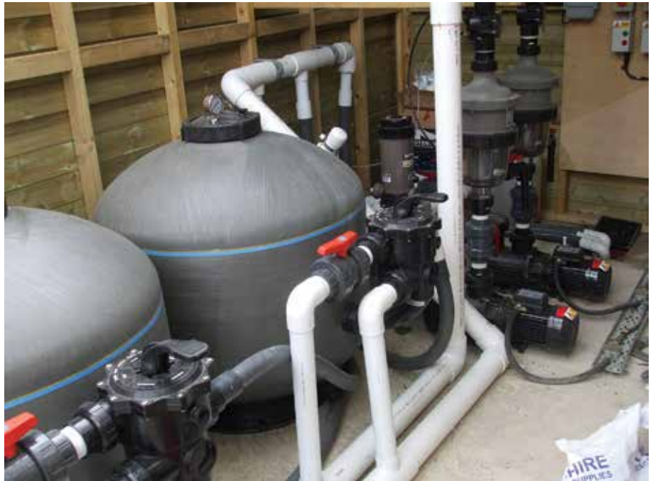
► Water is fed via two MultiCyclones and for extra clarity, the water was also fed through SM900 fibreglass filters filled with glass.
