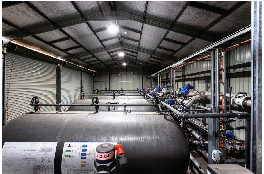
To deliver high-quality filtered drinking water free from unwanted taste and odours, Filtec installed Waterco's MPD10,000 Commercial Fibreglass Nozzle Plate Media Filter.
